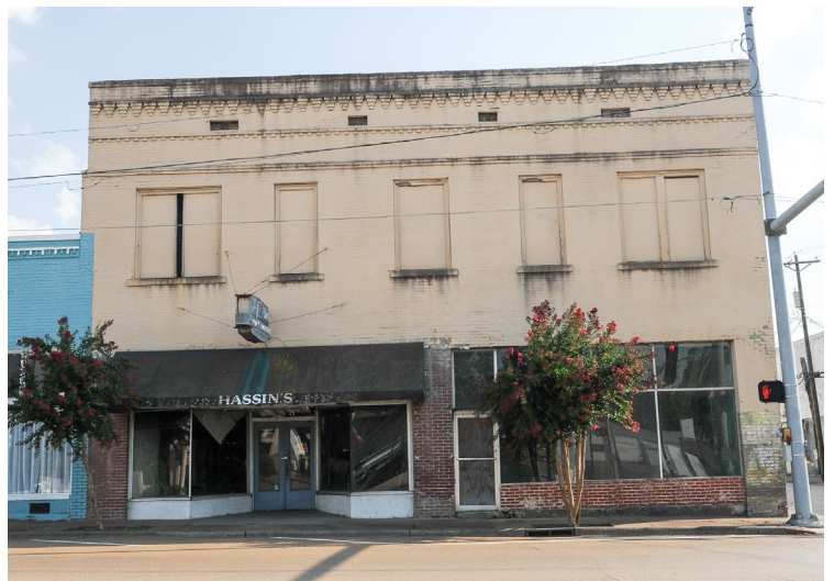
Properties in this type of condition do not allow for a potential tenant to open their business in the next 90 days. Property owners must make their properties tenable in order to recruit high quality tenants.
